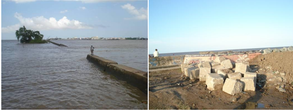
Guyana's sea walls and coastal defences are failing due to increased storms, coastal erosion, rise in sea level and lack of maintenance leading to increases in large scale flooding
