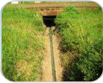
Most the latrines and sewers run directly into Lake Victoria
